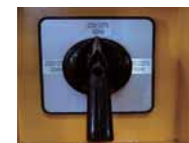
Multiple voltage selection on the panel
