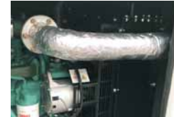
Safety Guard installed to protect inside from direct heat generated by exhaust and manifold
