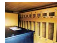
Perforated plate and rock wool within canopy
