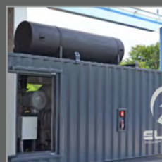
Residential Muffler on the roof it guarantees an acoustic reduction of the exhaust noise
